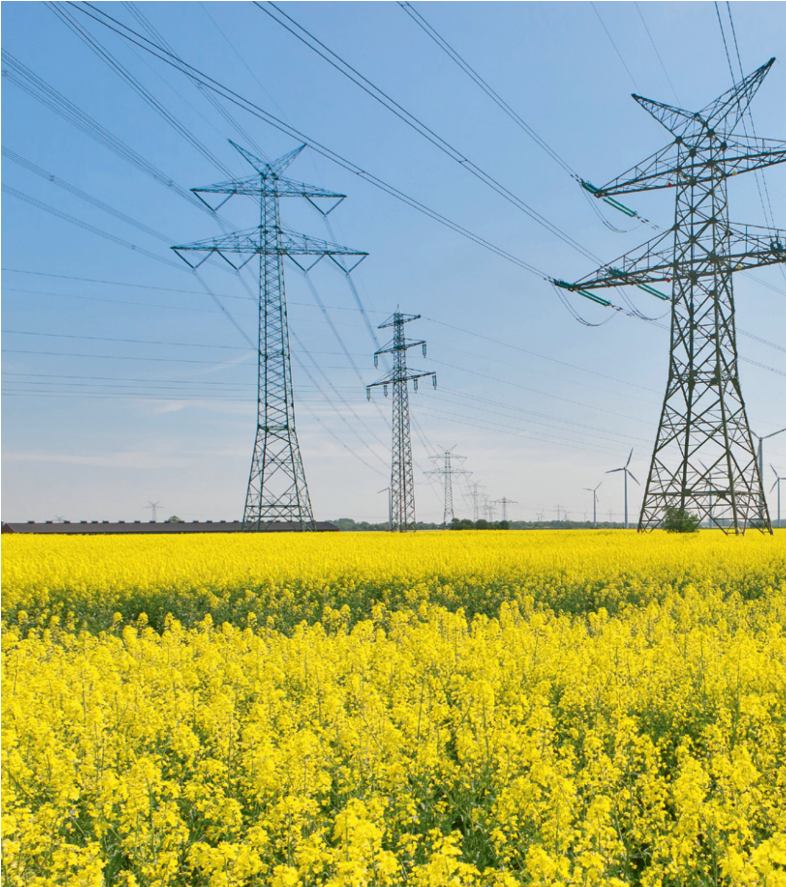
In Europe more than 6,000 kilometers of new power lines have to be deployed.
